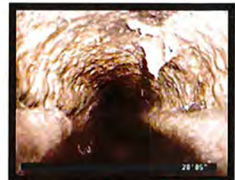
Clogged Sewer Line From FOG !
